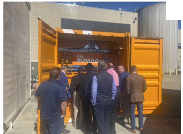
DUG's pod in Maryland
