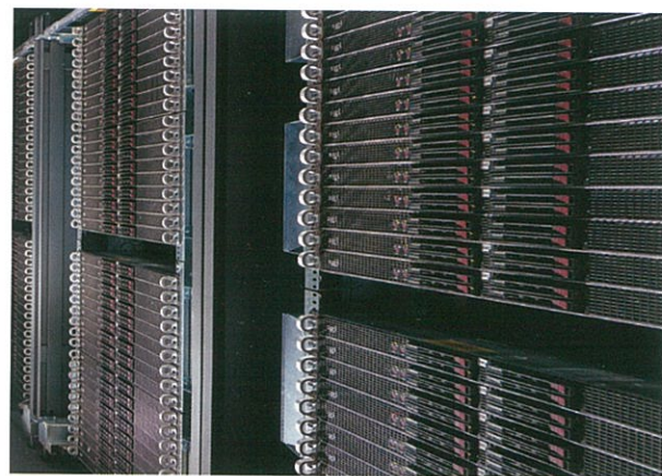
Storage and compute nodes in traditional water chilled racks.
