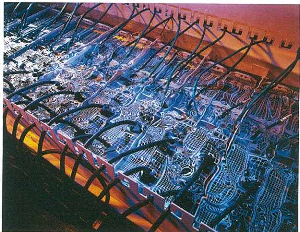
Compute nodes submerged in an oil bath. This saves up to 40% of the power costs.
